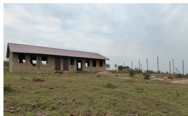
St. Lawrence Secondary first block with foundation for second block on right
